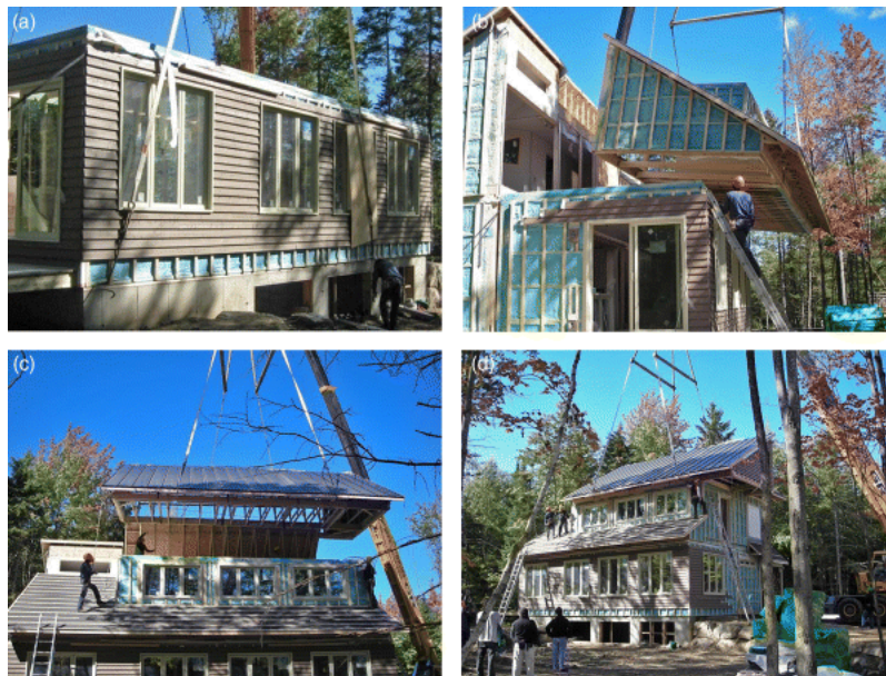
Fig. 7.3 Assembly of the ÉcoTerra house modules (a) main floor module; (b) lower roof section being lowered into place; (c) BIPV/T roof suspended above the second floor bedrooms; and, (d) all modules in place and connected
