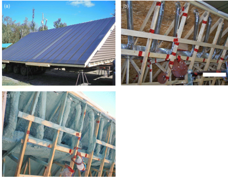
Fig. 7.6 BIPV/T roof: (a) finished roof module with PV modules attached; (b) underside of roof showing manifold (before insulation); and (c) underside of roof (insulated). Figures 7.6a and 7.6c reprinted with permission from Elsevier (Chen, Athienitis, and Galal, 2010a) © 2010, Elsevier
