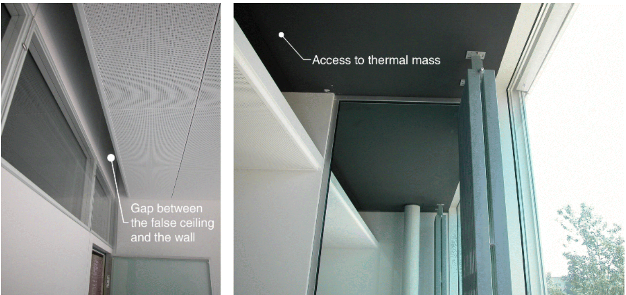
Fig. 4.6 Example of false ceiling that permits air circulation for thermal activation of concrete ceilings (BC-EPFL Lausanne Switzerland, Architect: R. Luscher Lausanne, Energy Concept: Sorane S.A, Ecublens)
