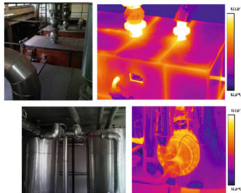
Fig. 4.12 Thermal images of case study building envelope and building service system elements
