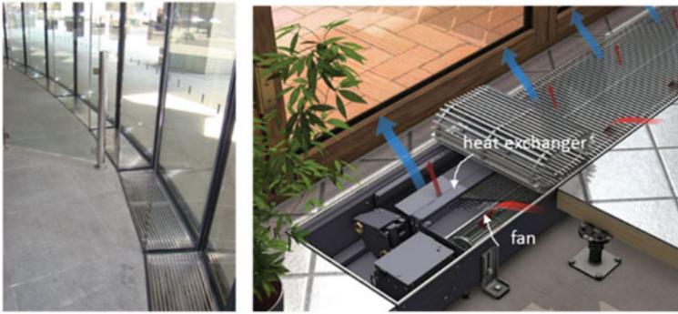
Fig. 8.19 Convectors installed into the floor below glass façade to compensate a cold air jet that descends from the glassing; draught is eliminated and thermal comfort is improved (left); (Bridge & PR Media Service Ltd.) forced convection fan-coil convector installed in a raised floor (right) (KI TDC d.o.o.)
