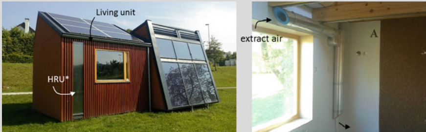
Fig. 11.32 HRU* is integrated into south-orientated wall and has a transparent cover to utilize solar energy by additional heating of the fresh supply air; in the present calculation, only heat transfer between the exhaust and fresh air is taken into account
