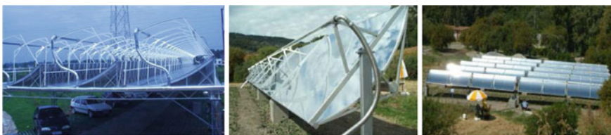
Fig. 9.10 Parabolic CSC with area 32 m 2 that drives double stage absorption chiller with rated cooling power of 16 kW (left), (Broad Technology Centre, China) 180 m 2 CSC array of the double-stage chiller with cooling power of 116 kW [middle, right; Lokurly 2010]
