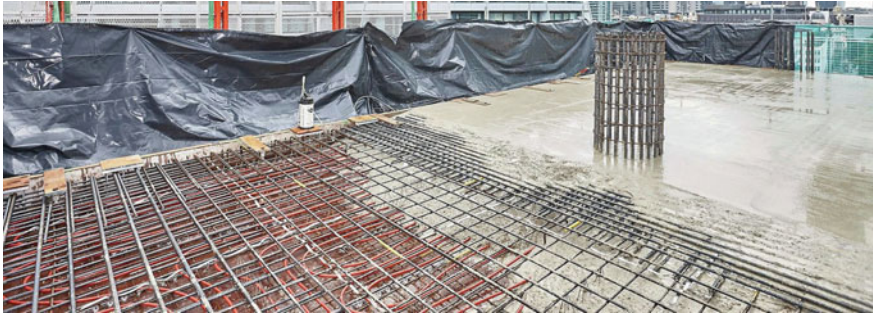
Fig. 8.31 Pipes built-in in the core of the concrete-bearing plate in office building; circulation pipes must be installed in TABS during the construction of the building ( www.rehau.com )
