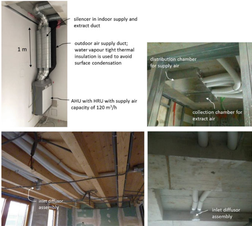
Fig. 11.27 Octopus type of distribution duct system in apartment; each tube has diameter of 80 mm and air flow rate is designed to 30–40 m 3 /h per duct; this corresponds to the physiological needs of one person. If two persons are expected to be in the room, two ducts are connected to the assembly of inlet diffuser
