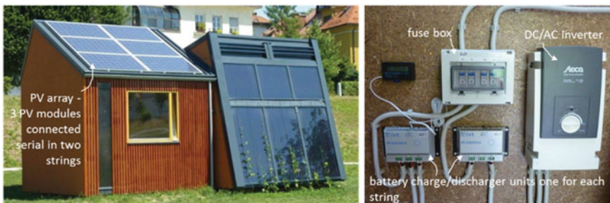
Fig. 7.13 Off-grid PV system installed on the virtual lab building
