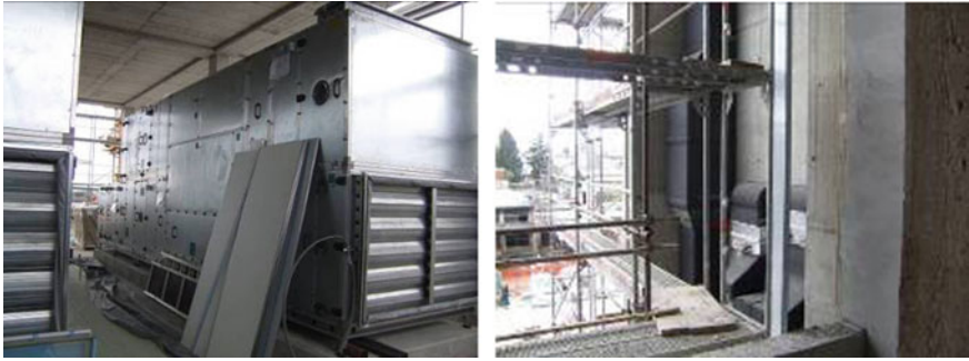
Fig. 8.23 AHU on the roof of the office building (left); vertical channels for supply of ventilation air (right)
