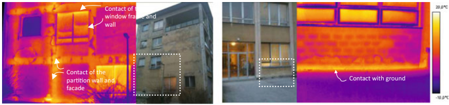
Fig. 3.10 During the period of low external temperatures and heating period, heat bridges can be detected by thermal imaging; typical thermal bridges in non-thermal insulated buildings are presented on the photos
