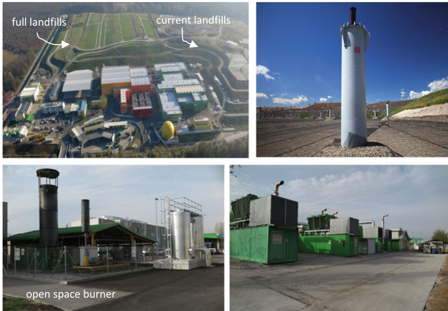
Fig. 2.22 Centre for solid waste treatment of Municipality of Ljubljana that will replace landfills in the future (top, left); landfill ready for municipal solid waste disposal with water-tight membrane and set of degassing shafts (top, right); landfill gas pumping station with open burners where landfill gas is burned if the content of methane in the landfill gas is lower than 40% or during the maintenance (bottom, left); system of landfill gas power plants as cogeneration units; unit can produce electricity and heat if the amount of methane in landfill gas is above half of designed value (bottom, right) (Trivunčević 2016)
