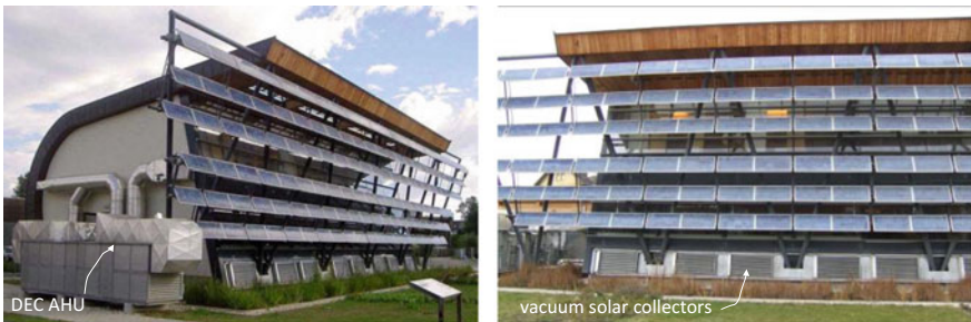
Fig. 9.31 DEC solar cooling system for space cooling of office building; AHU has rated capacity of 6000 m 3 /h and rated DEC cooling power is 30 kWc; heat for dehumidification of the desiccant wheel is delivered by vacuum solar collectors array with area of 12 m 2 ; DEC system produce 10,000 kWh of cold at seasonal coefficient of performance 0.6 . ( www.oekoplan-hartberg.at )
