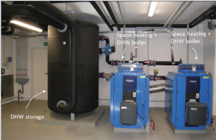
Fig. 10.5 Space heating and DHW boiler in a multifamily building
