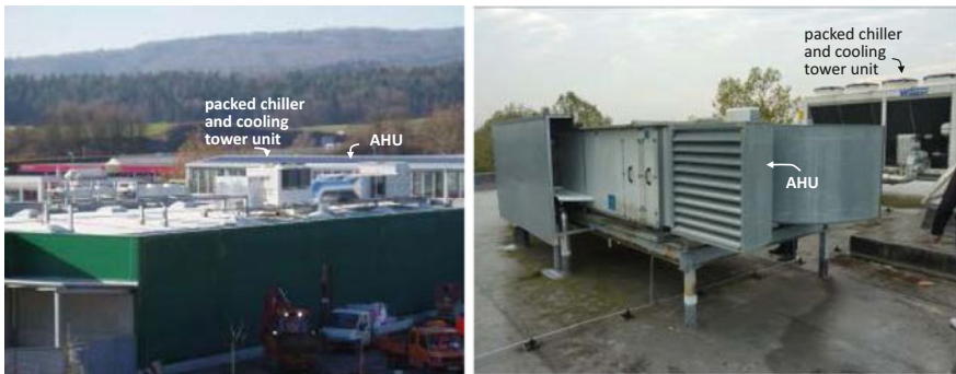
Fig. 9.15 Packed chiller and cooling tower unit on the top of the roof of shopping centre (left) and office building (right). To prevent freezing of water in the outdoor section of a chilled water loop (i) antifreeze fluid (glycol) could be added to chilled water, (ii) pipeline could be heated by a wire electrical resistance heater installed on the pipes’ outer surface, (iii) a chilled water pipeline can be drained manually until next cooling season
