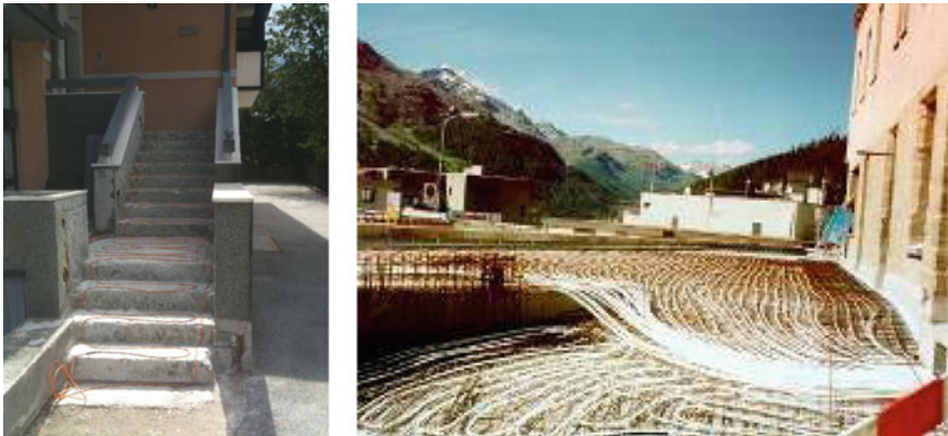
Fig. 8.32 Stairs heated with electrical resistant heater (left); ground heating of pavement in St. Moritz; in this case, heating water must be mixed with antifreeze fluid (right)
