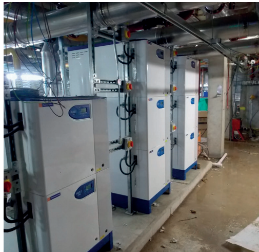
Figure 8.15 Insulated Heat interface unit (HIU) in dwelling (left).
