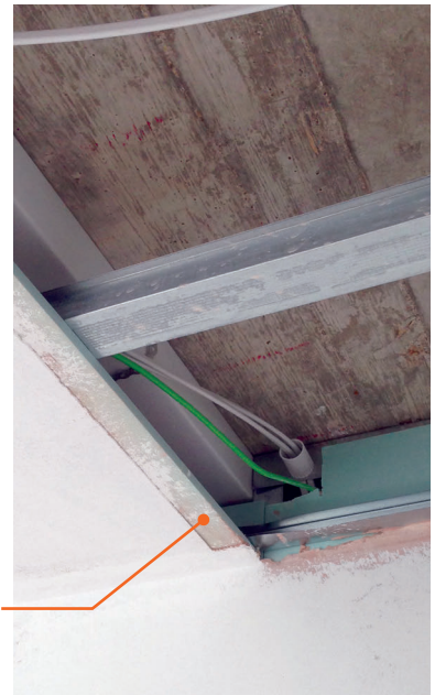
Figure 4.19 Concrete soffit with suspended ceiling zone for services and layer of mineral wool. A deeper ceiling zone with space for circular duct will improve performance of ventilation system.
