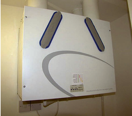
Figure 8.34 MVHR installed in cupboard (bottom left).
