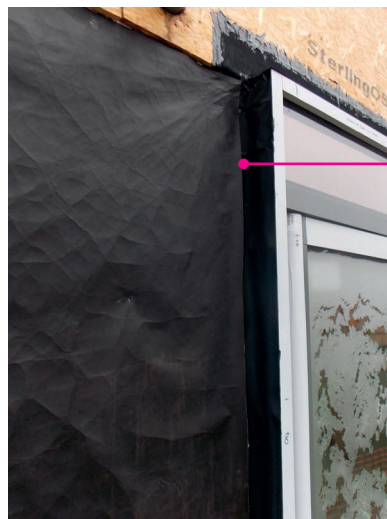
Figure 7.10 Window head and jamb with cavity closer and thermally separate lintel (left).
