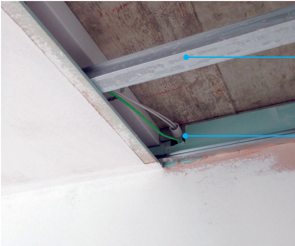
Figure 8.47 Gaps in insulation layer cause extra heat loss. Penetrations in external envelope need to be cut accurately, with no gaps in insulation.
