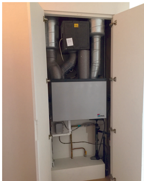
Figure 8.2 Typical services cupboard or utility room in a home (left).
