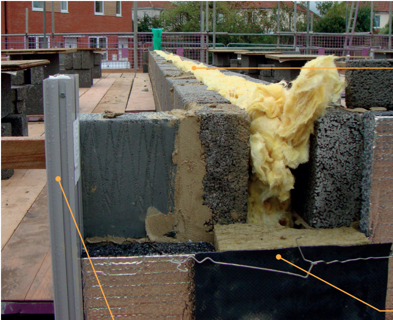
Figure 3.23 Party wall between two houses with entrance door tight either side can be tricky to build.
