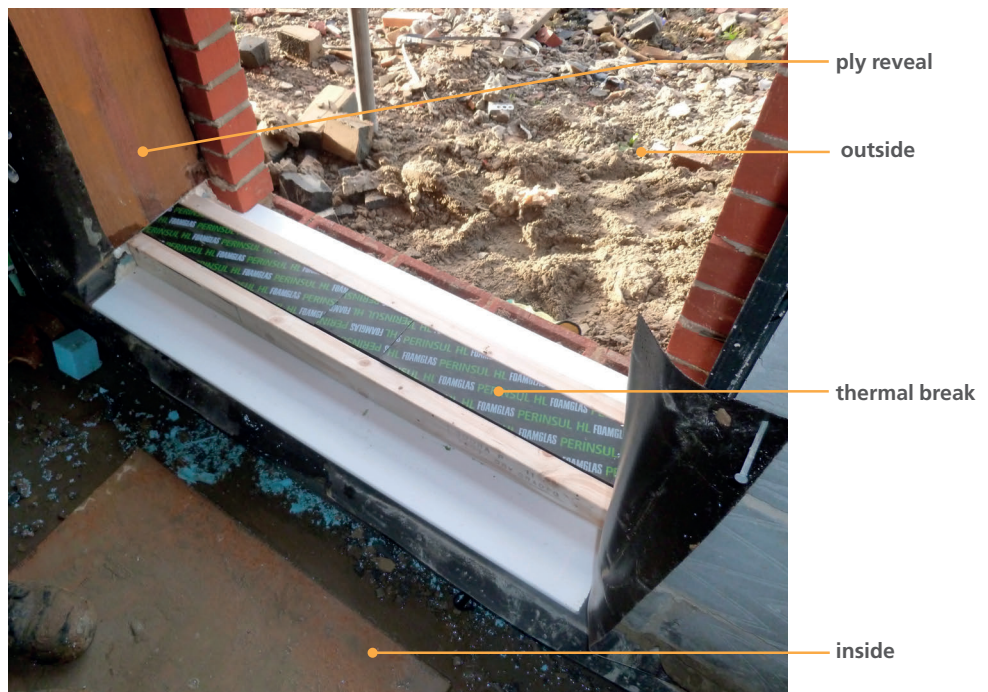
Figure 3.15 Level threshold detail showing thermal break and temporary timber batten as protection.
