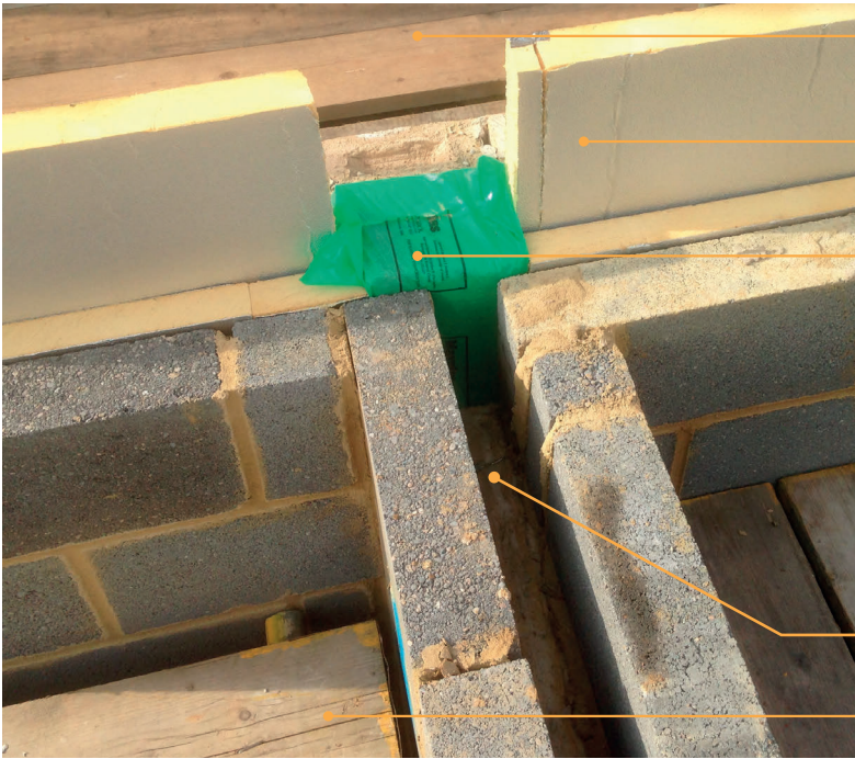
Figure 3.24 Party wall and external wall junction from above – rigid insulation on external wall requires a separate fire barrier / edge seal.
