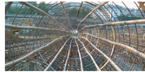
Fig. C2.31 Drilling pile during construction of a building. By layering the pile with pipelines, an energy pile for heating and cooling may be created.
