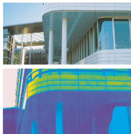
Fig. C3.3 Infrared imaging shows that the supports penetration of an overhanging ceiling does not cause thermal bridges
